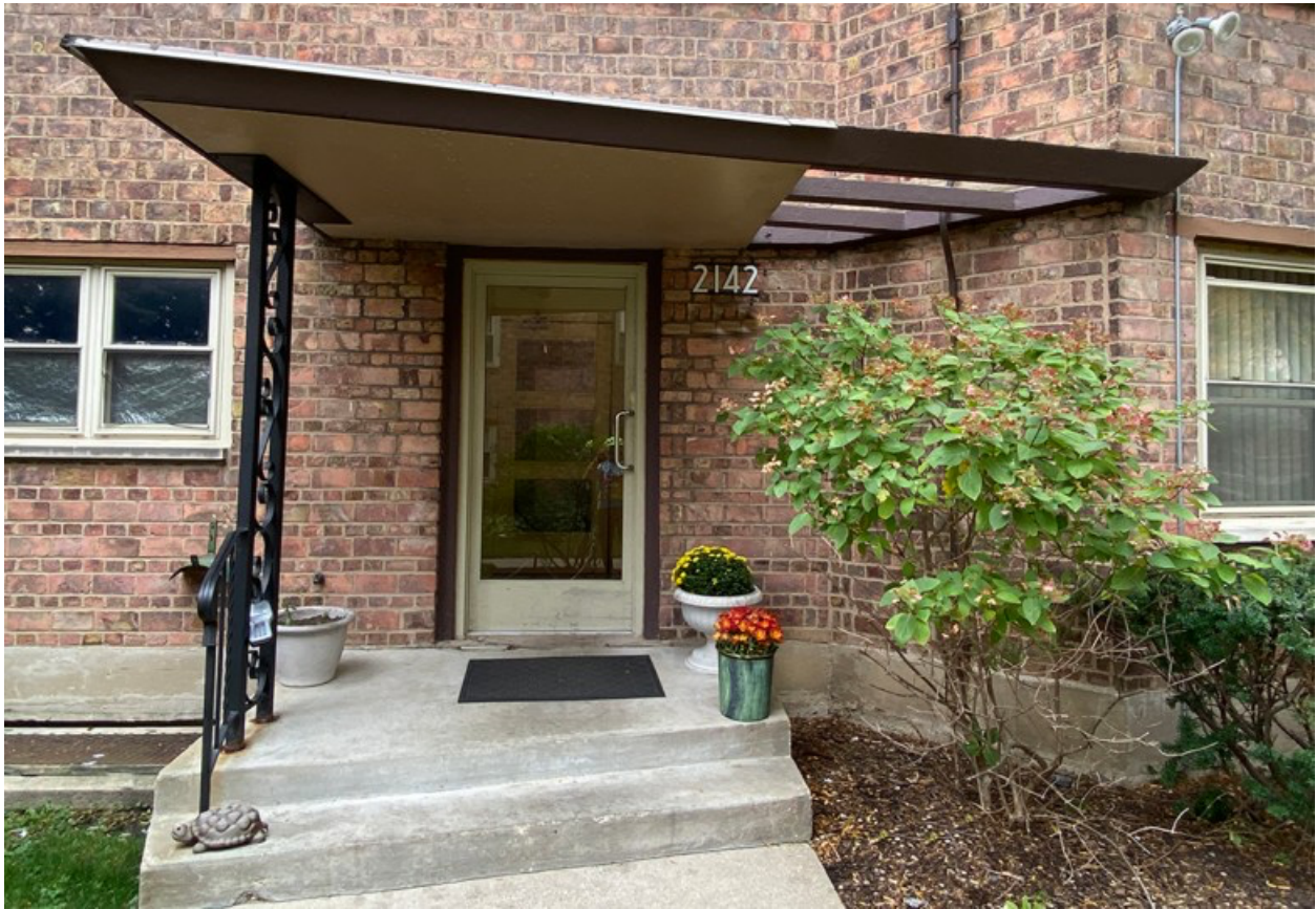
The entrance canopy at 2142 W. Rosemont Ave. is punctured with openings to allow light over the entry door. Credit: Jack Weiss
